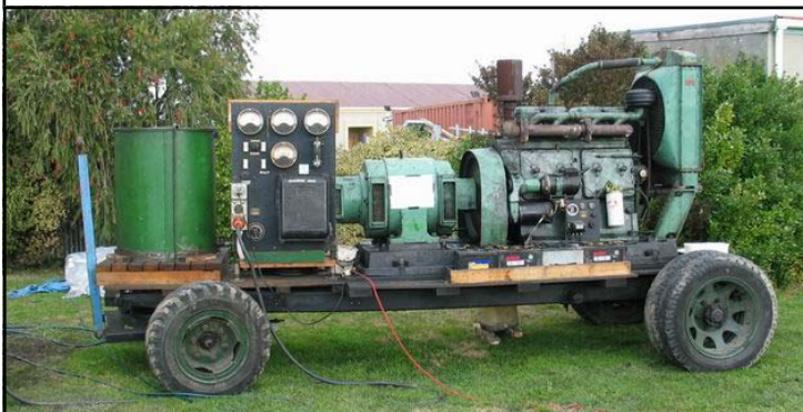
Lister Diesel Generating Plant
